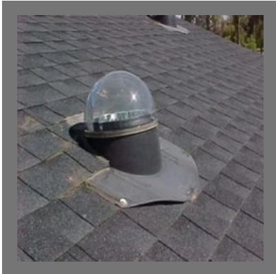
Rooftop Tubular Skylight
